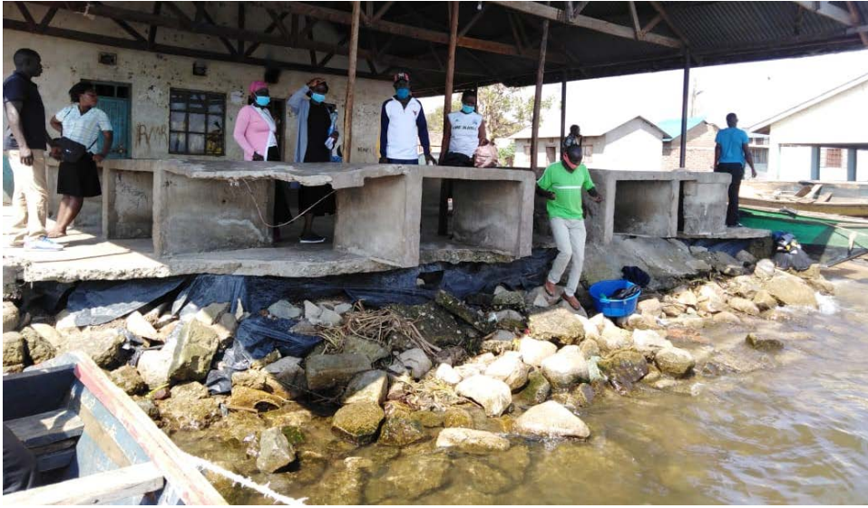
Plate 9: Nile perch receiving slabs destroyed by rising water level in Kenya
