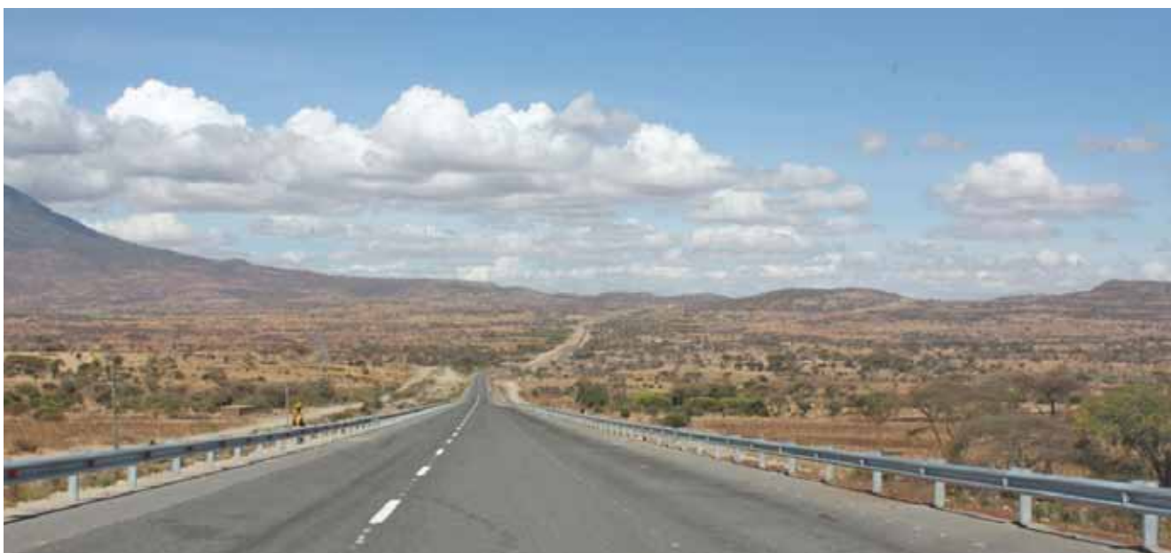
A section of the Arusha-Namanga-Athi river road. Inter-connectivity is key for economic growth of the region
