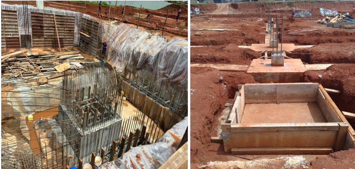
Photo showing the status of basement and ground floor (main hall). Taken by Audit Commission on 20 November 2023.
